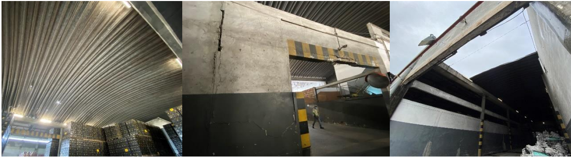
Figure 5: Finished Goods Warehouse – Anomalies
