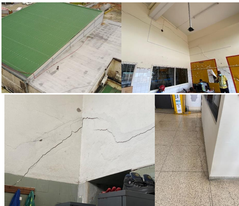
Figure 3: Laboratory / Technical Building – Anomalies
