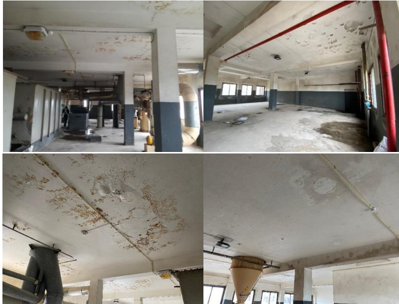
Figure 8: Silos Building – Anomalies
