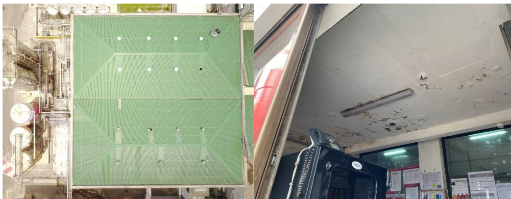
Figure 2: Canteen and Filtration – Anomalies
