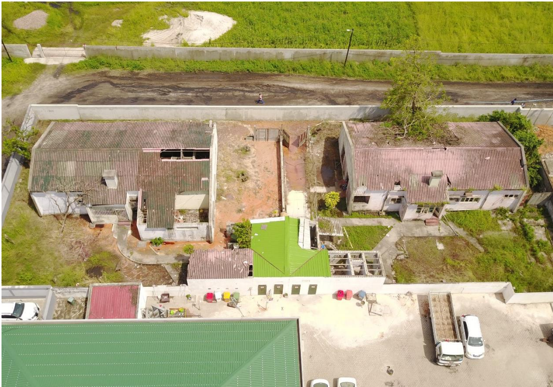
60. Residences: roofs in advance state of degradation
