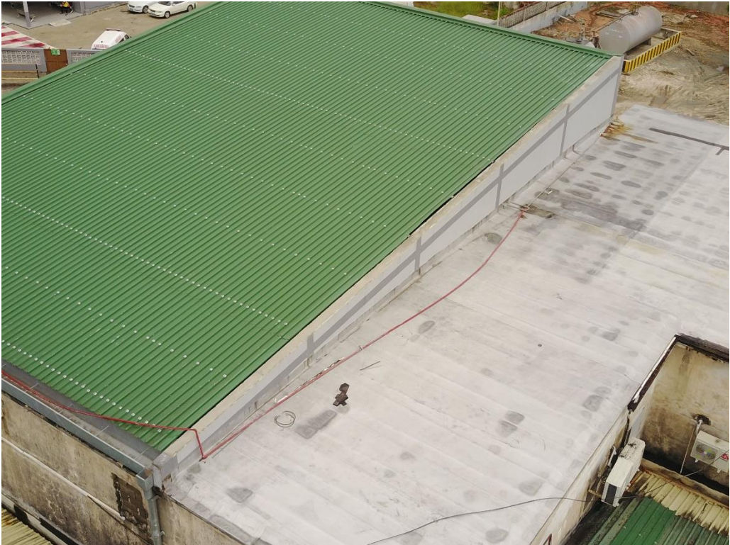
18. Laboratory and Technical Building: no flashing
