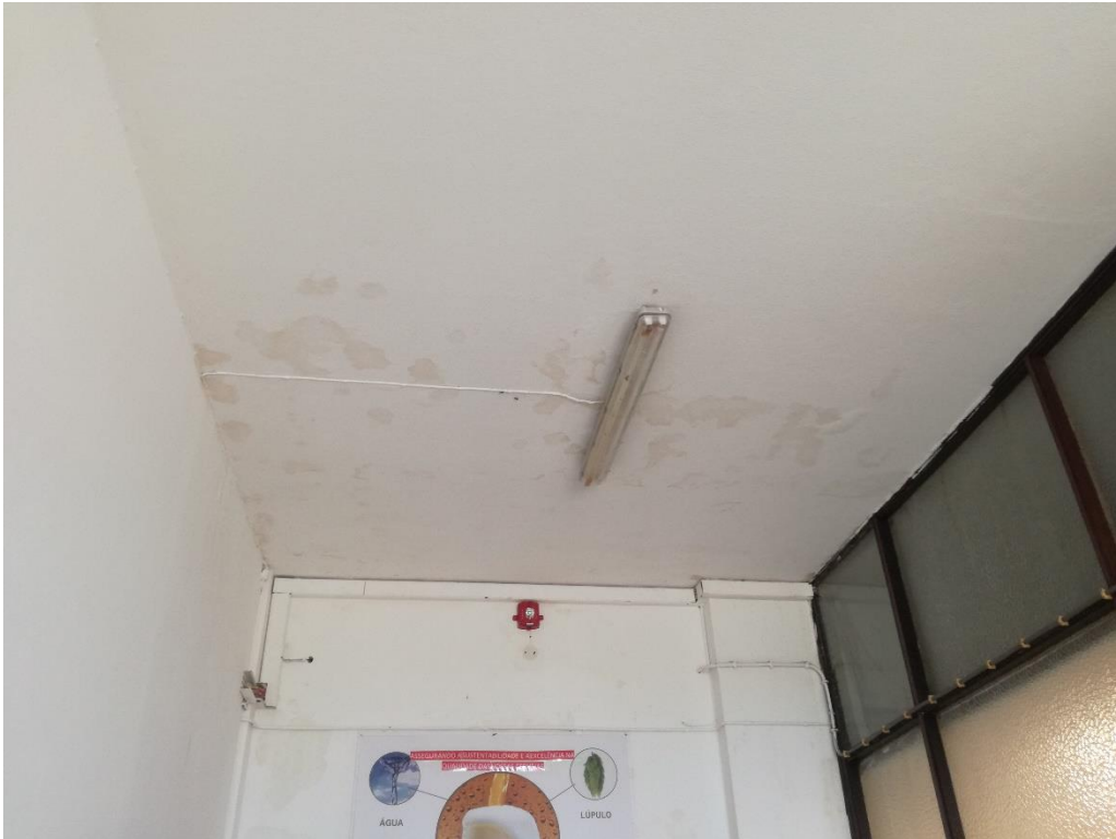
19. Laboratory and Technical Building: water infiltration in the slab soffit
