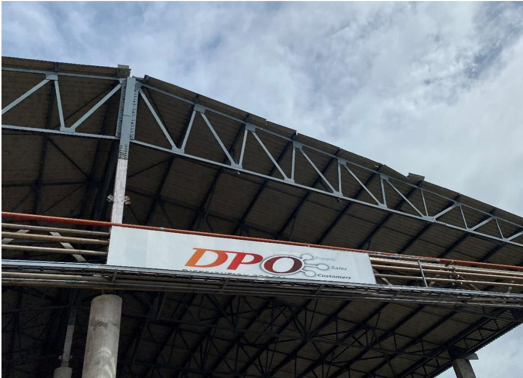
41. Un/Loading Bay – North: new roof with torn sheets at the end and missing ridge cap
