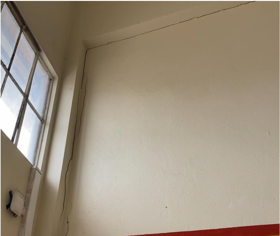
22. Laboratory and Technical Building: large cracks in the walls
