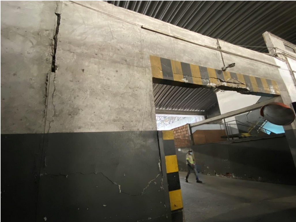
39. Finished Goods Warehouse: cracks in the beam and wall
