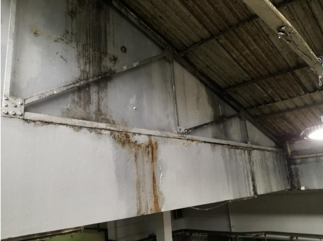
30. Pack Hall: Water Infiltration Due to Defective Waterproofing
