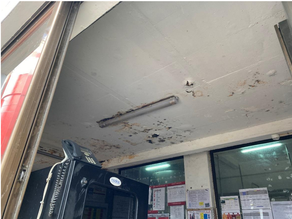
16. Canteen and Filtration: water infiltration on the slab soffit of filtration room
