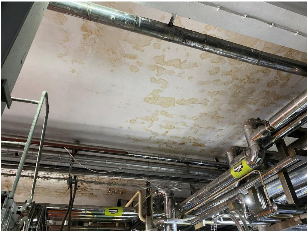
56. Engine Room: water infiltration in the ceiling
