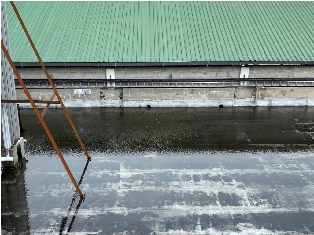
57. Engine Room: roof slab with inefficient drainage system
