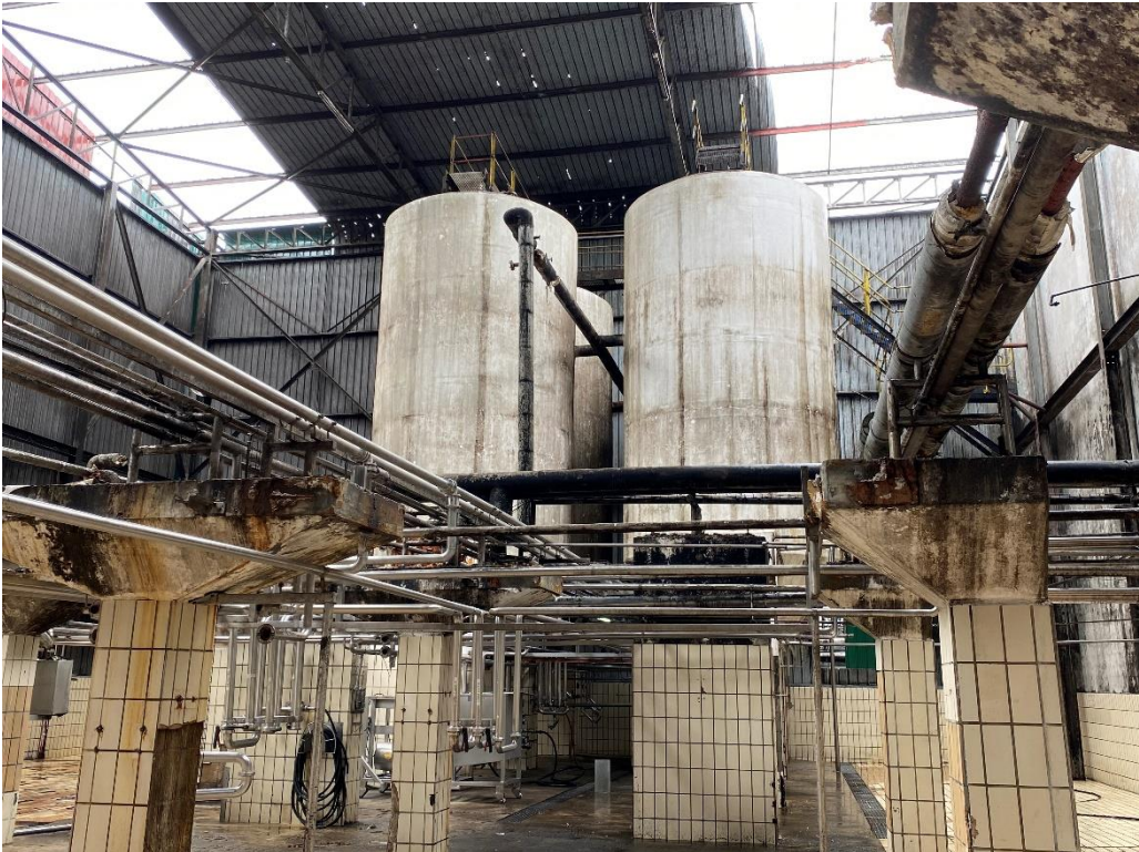
11. Old Cellars: view inside the building showing the damages in the supporting structures
