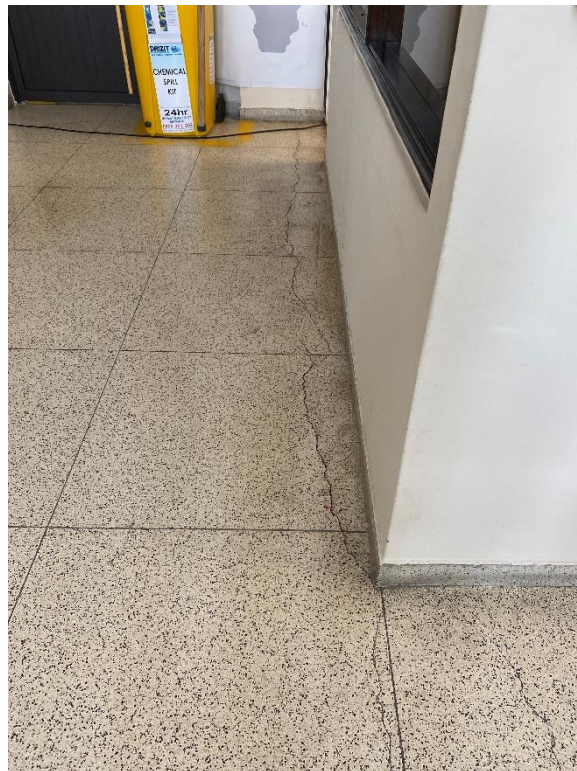
24. Laboratory and Technical Building: large cracks in the floor
