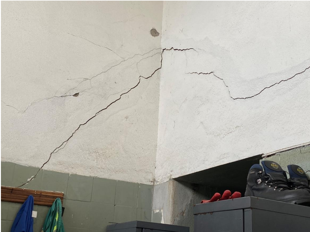
23. Laboratory and Technical Building: large cracks in the walls
