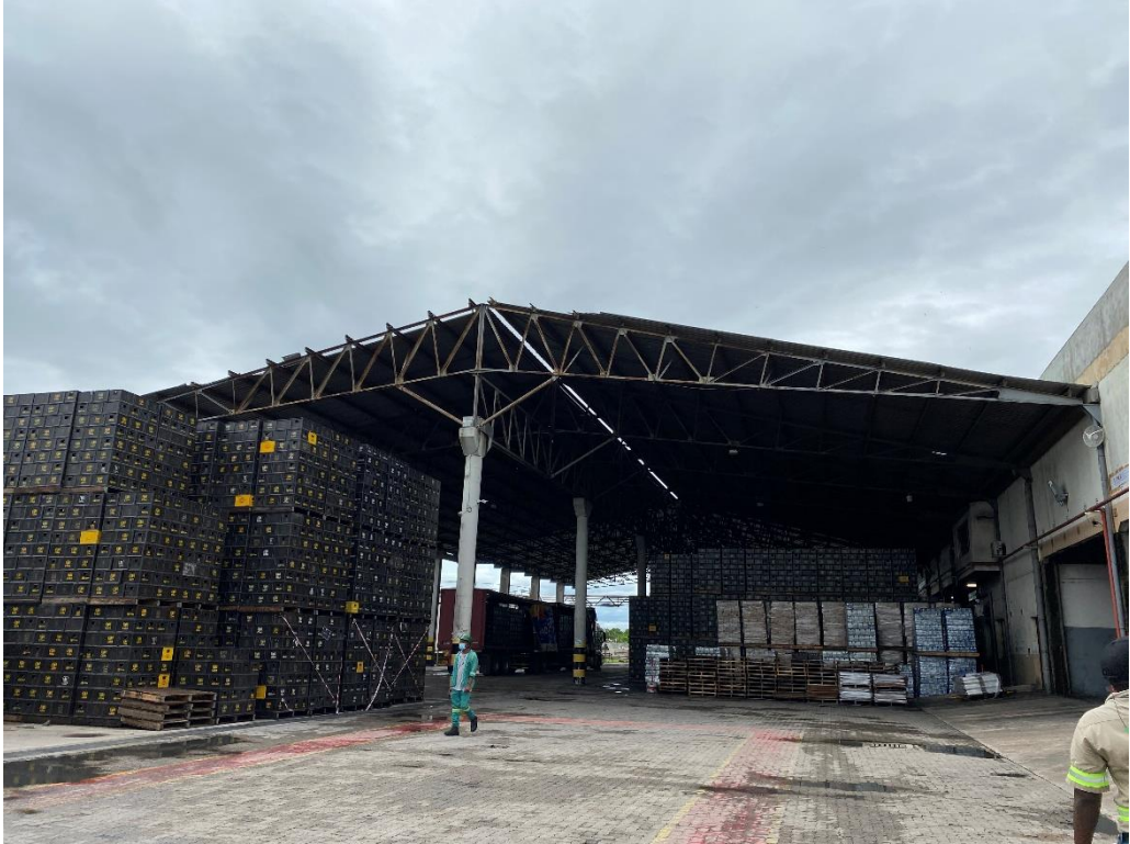
42. Un/Loading Bay – South: roof missing the ridge, torn sheets and corroded roof structure
