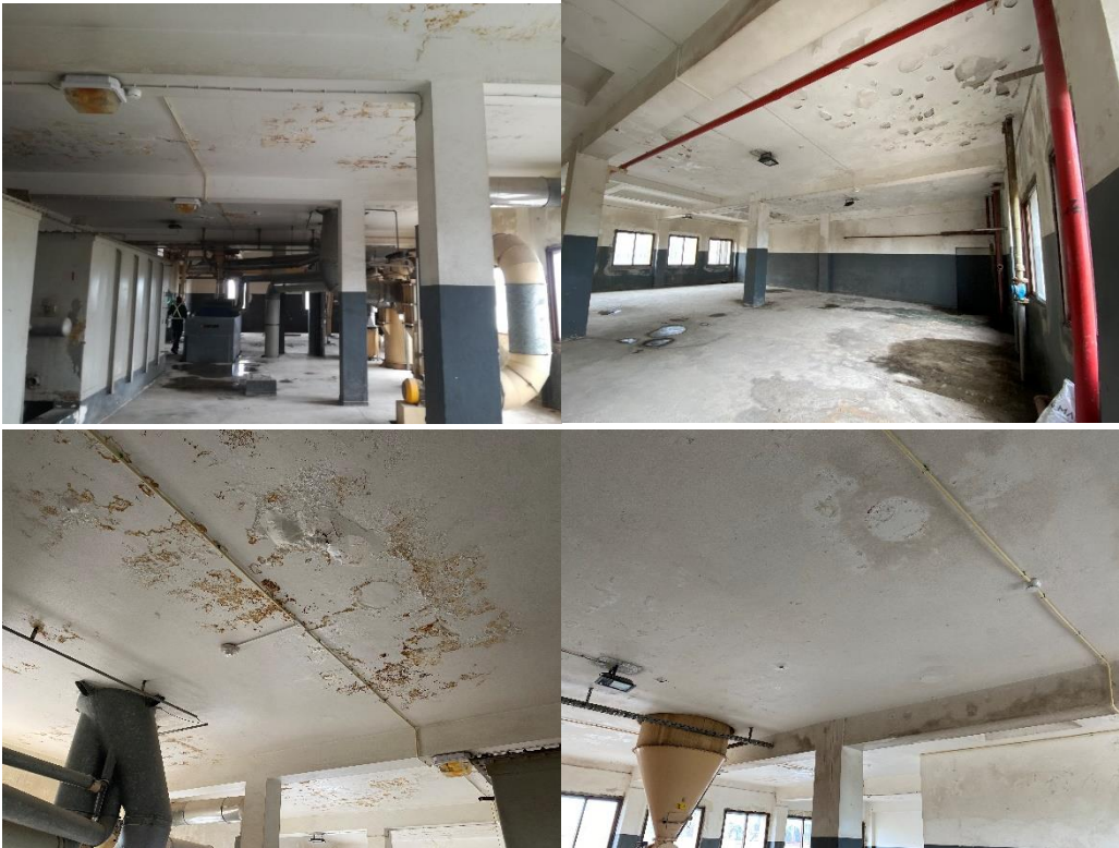
52. Silos Building: water infiltration in the slab soffit (different floors)
