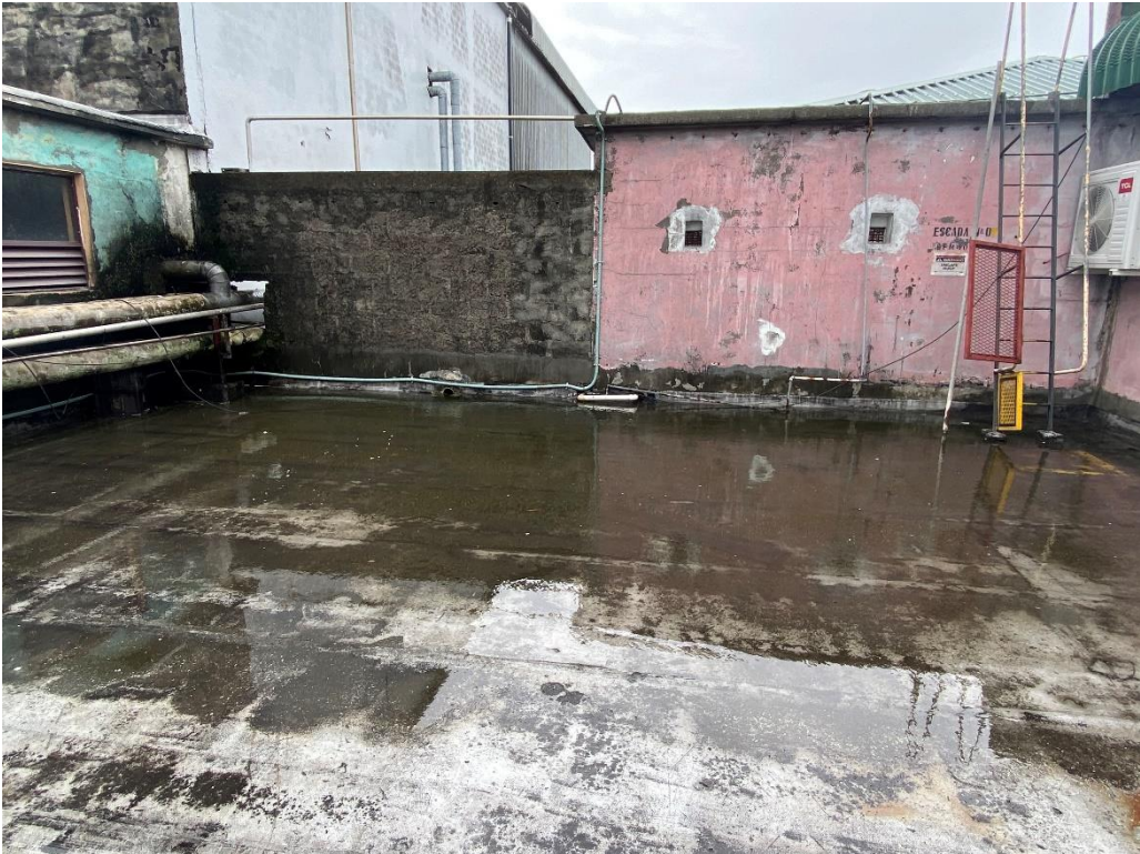
29. Pack Hall: poor drainage system on the roof slab
