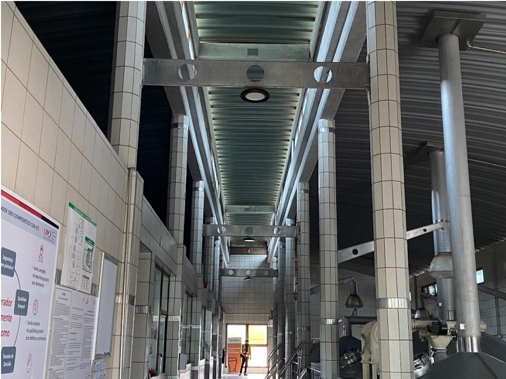
7. Brew House: damaged concrete columns
