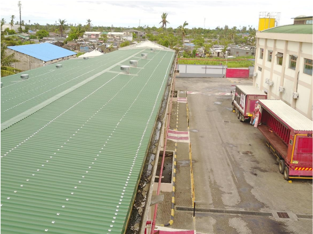
50. Raw Materials Warehouse: concrete gutter in poor condition
