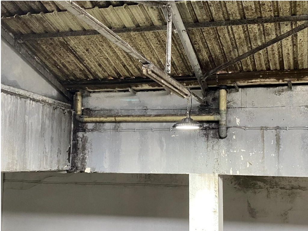
31. Pack Hall: gutter in degrading condition
