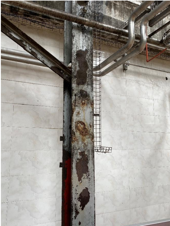
13. Old Cellars: structural column with advanced state of corrosion
