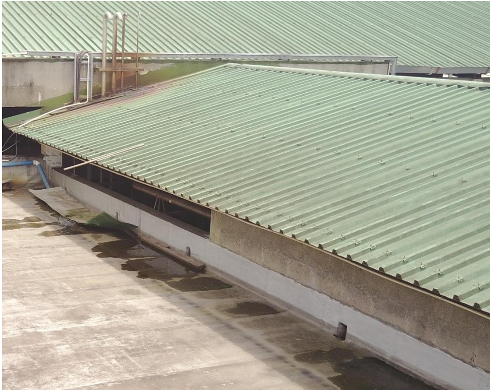
53. CO 2 Plant: opening that allows rainwater inside the building
