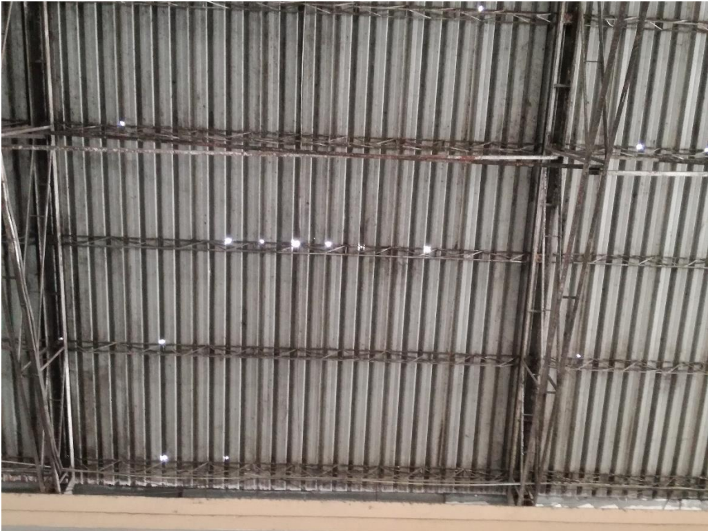
35. Pack Hall: roof with signs of corrosion
