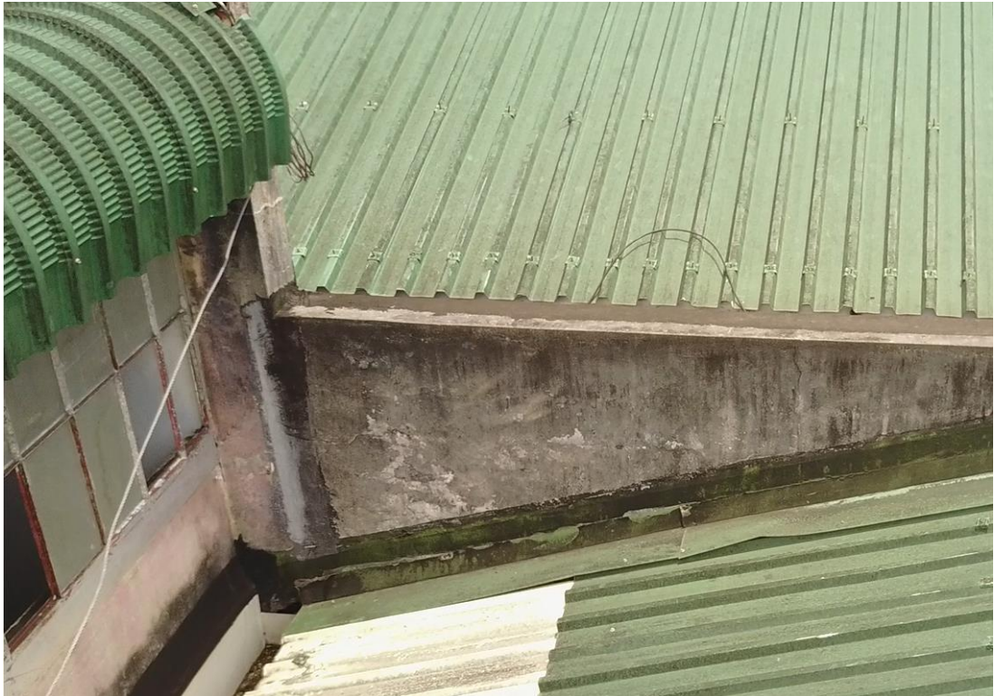
27. Pack Hall: gutter and waterproofing in poor condition
