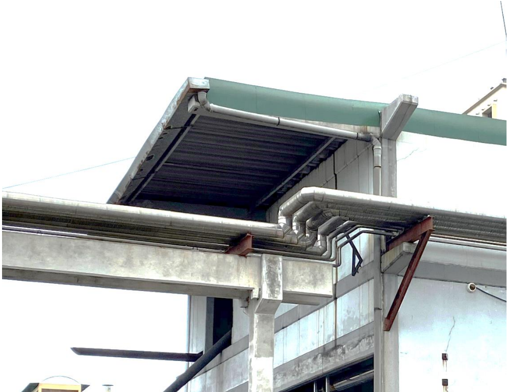
59. Boilers: corrosion in gutter and roof
