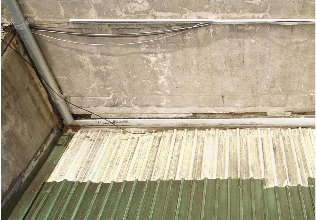
26. Pack Hall: gutter and waterproofing in poor condition
