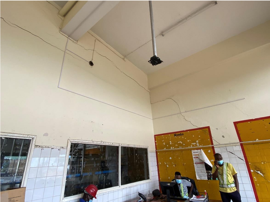
21. Laboratory and Technical Building: large cracks in the walls
